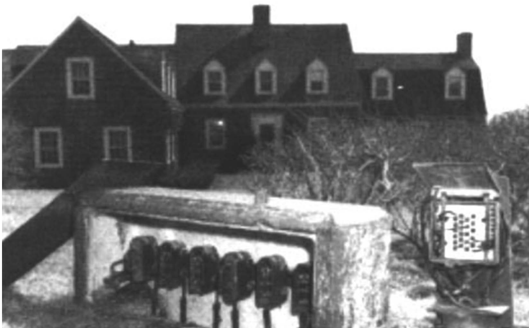
Figure 3. The first underground residential distribution (URD) cable system was based on rubber cable operating at 5 kV (Fishers Island, NY.)
